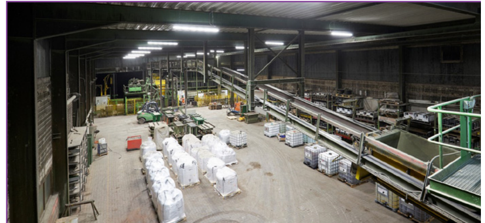
Ensuring the best working conditions at our operations is vital. Minimising our energy usage is also a core focus. In 2019, a supplier was identified to scope and install a LED scheme at the EHL Rossla plant, part of our Building Products Division in Germany. The installation of this LED technology has resulted in a decrease in energy usage of over 97,000 kWh at the Rossla plant, as well as significantly improving safety and working environment standards across the site.
