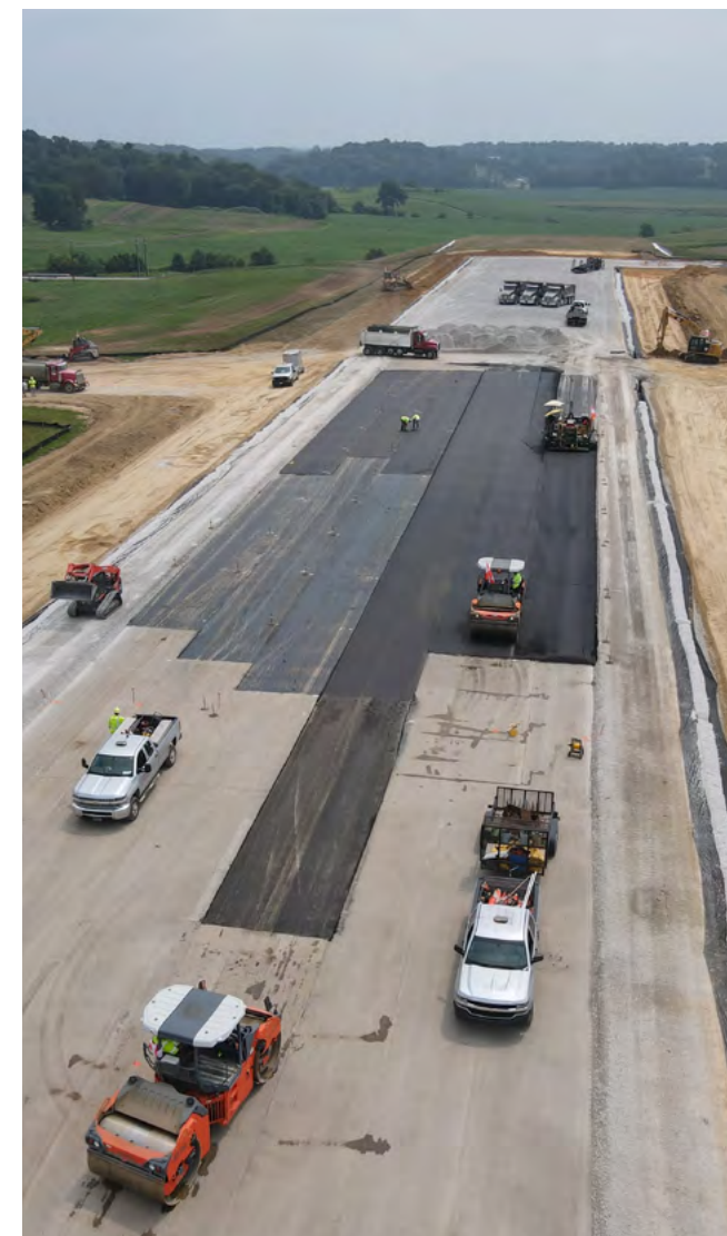
J.H. Rudolph & Co., Inc, part of CRH's America's Materials Division, delivered this runway extension project at Huntington Regional Airport in Indiana, United States. The project included increasing the length of the runway by over 500 feet and the construction of Indiana's first traffic tunnel under an airport runway.
