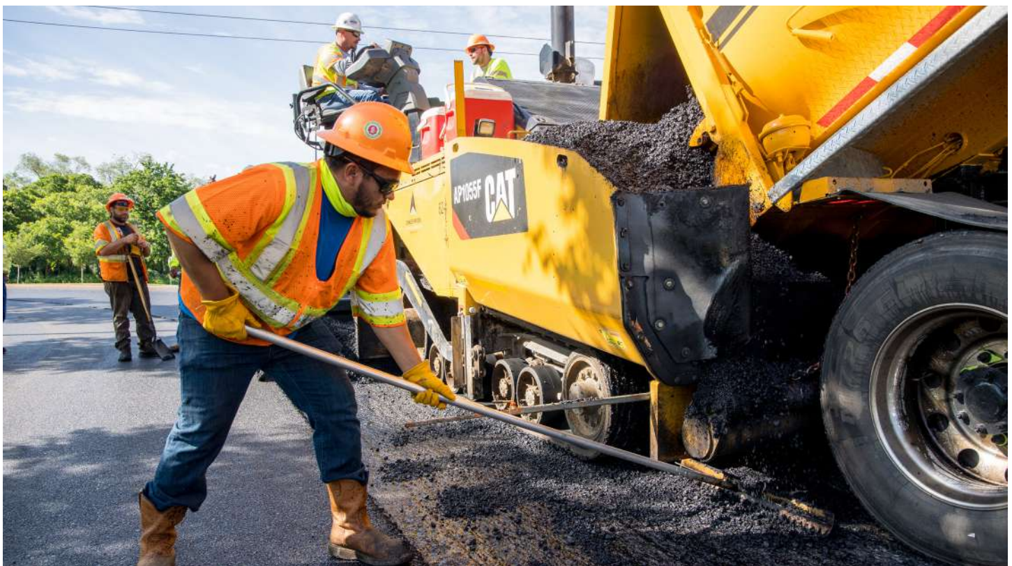
Staker Parson Materials & Construction, part of CRH's Americas Materials Division is a leading provider of paving, concrete, construction services and landscaping in Utah. CRH is the largest producer of asphalt in North America. The material is 100% recyclable which helps make CRH a significant contributor to the circular economy.
