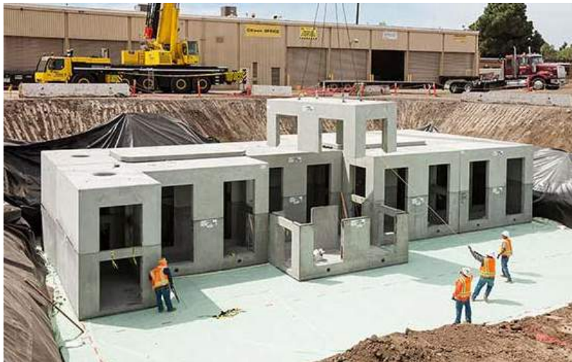
The Metro Expo Light Rail operations and maintenance facility in Santa Monica, California, US, uses Storm-Capture units to harvest and store rainwater for reuse in landscape irrigation and vehicle washing. Oldcastle Stormwater Solutions, part of Oldcastle Precast, was involved in the design and construction of a concrete stormwater management system to reduce the impact on the municipal water supply in this high drought area.
