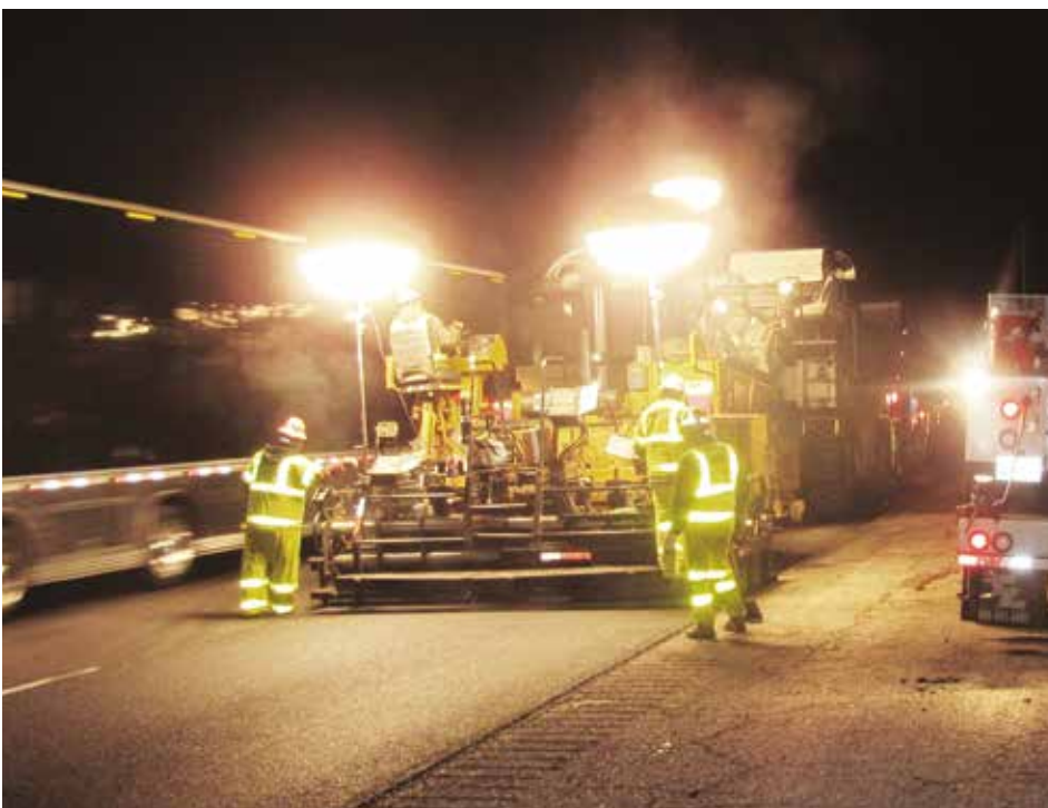
The "AWARE" system is a new innovative safety technology being trialled at Oldcastle Materials, US. It increases the safety of employees and contractors by alerting them to work zone intrusions by third party vehicles that could result in serious accidents and fatalities.
