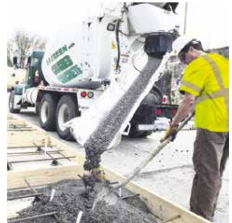
Harrison Construction, which has operations in Tennessee and North Carolina, US, has invested in an award-winning mobile crushing operation to recycle and reuse materials that would otherwise be discarded, increasing the sustainability of its products and business.
