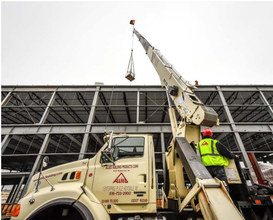
Allied Building Products delivering the PVC Roofing System for the new 500,000 square foot Fresh Direct distribution centre and corporate headquarters at the Harlem River Yards in the South Bronx, New York.
