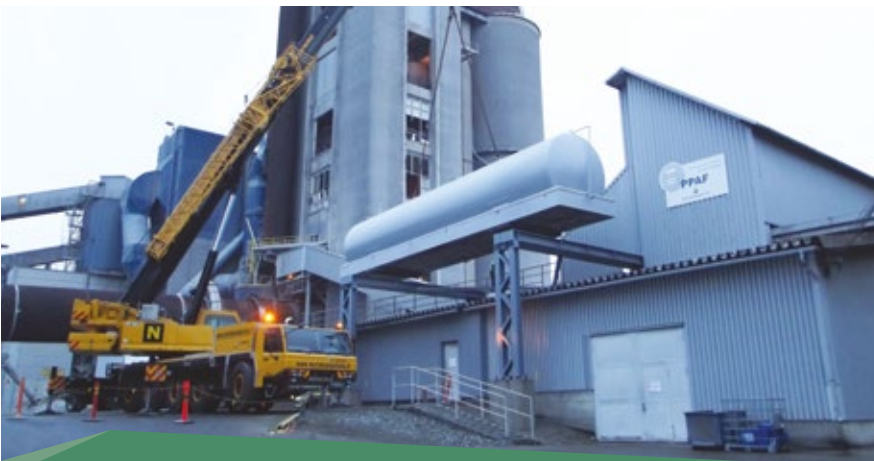
Finnsementti installed a new water tank as part of its water management system at its Parainen cement plant in Finland.
