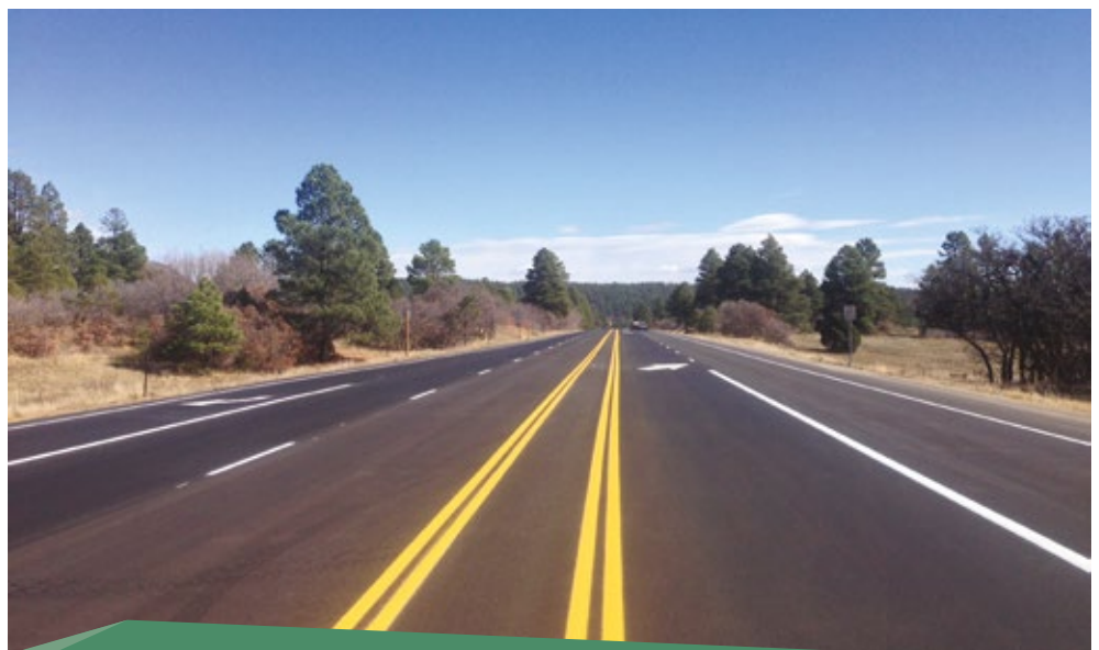
Four Corners Materials, received an award from the Colorado Asphalt Pavement Association for work on US Highway 160. The award-winning project, located in southwestern Colorado, consisted of resurfacing 10.2 miles of three-lane roadway. This amounted to 52,000 tons of asphalt with 20 percent recycled asphalt pavement.
