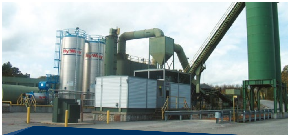
The asphalt plant in Westbrook, Maine, US, purchased from Lane Construction in September 2014 by Pike Industries. The plant, which is fired on natural gas, includes equipment to enable the use of recycled asphalt pavement.
