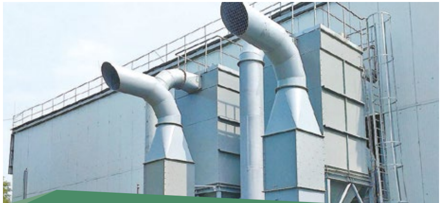
Mykolaiv Cement, Ukraine, has installed and commissioned a new clinker intake facility.
