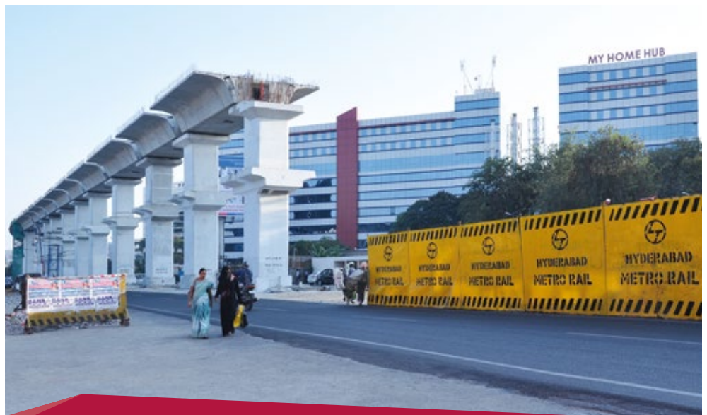
Concrete for a new major metro line in Hyderabad, India is provided by My Home Industries Limited, a CRH joint venture.
