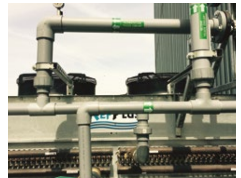
There is a focus on energy at Oldcastle Precast's Candiac location in Quebec, Canada, where all electricity purchased is generated from renewable sources and a heat recuperation system was installed during 2014 to improve energy efficiency.
