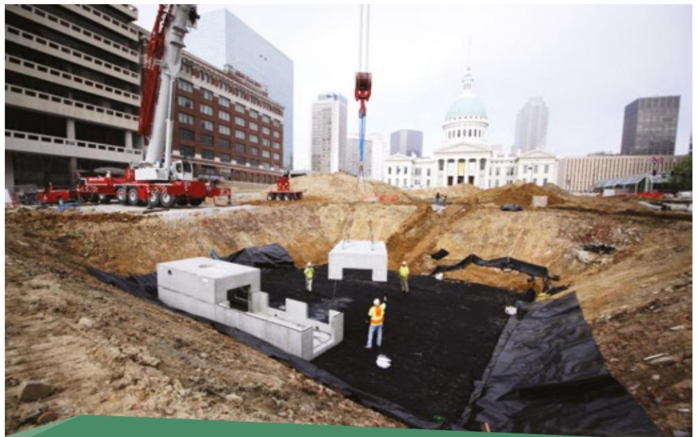
Oldcastle Precast, which operates throughout the US, offers a variety of solutions for stormwater management needs that assist with control of runoff, prevention of storm drain overloading and other downstream issues such as flooding. Pictured is a system being installed at the City River Arch project in St. Louis, Missouri.
